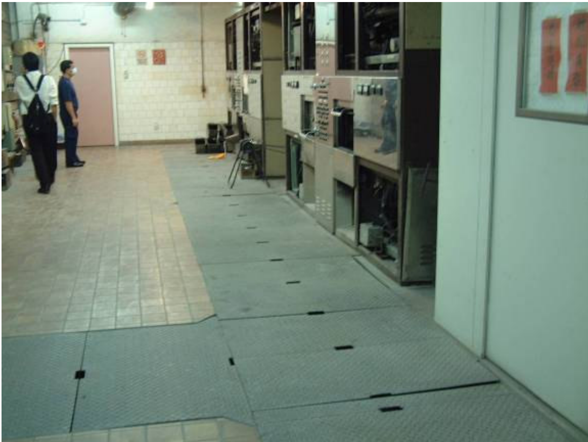
Photo 5 – Interior of Coffin Crematorium and Area with Sunken Fuel Pipe
