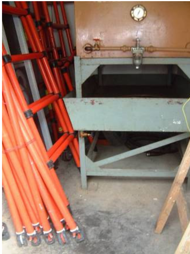
Photo 11 – Day Tank Room
