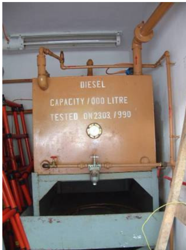
Photo 10 – Day Tank Room
